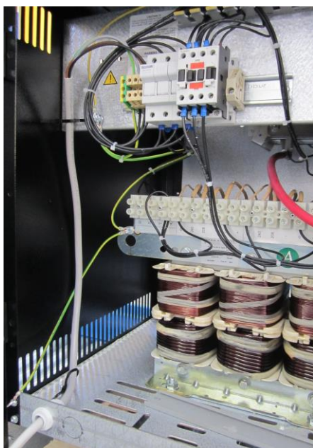
This Picture shows how mains connection to LP cabinets is performed
